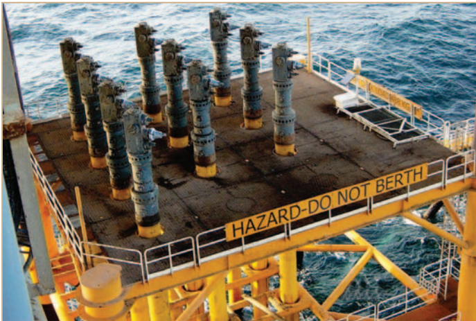
A completed well with the external valves removed awaiting stab over of the topsides facilities.
